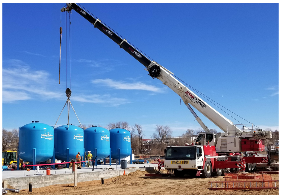
Ion Exchange vessels used to treat PFAS were recently delivered to the site of the new water treatment plant.
